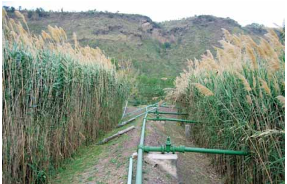
A Root Zone Biotech plant at ACC Gagal that enables treatment and recycling of waste water.
