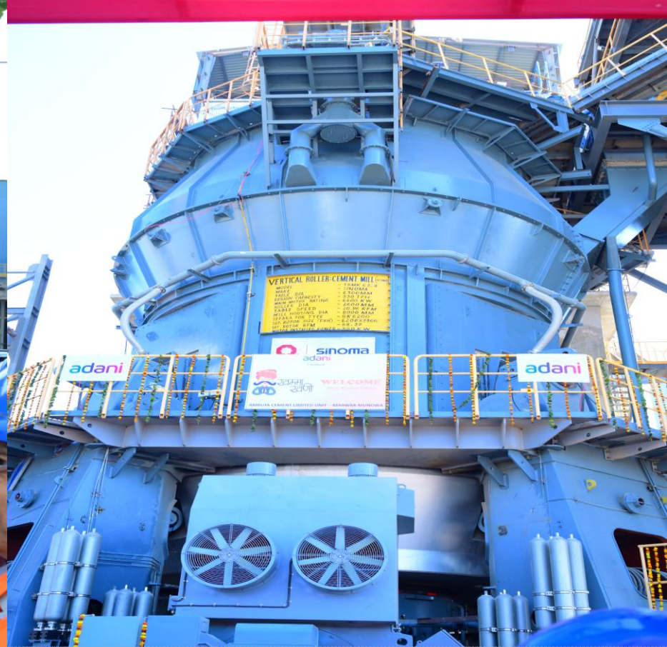
Marwar Vertical Roller Cement Mill
