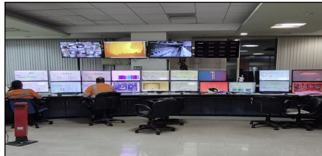
Central Control Room (CCR) The CCR is the plant's digital hub, continuously monitoring and optimizing all key processes
